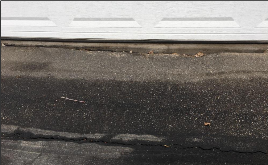
Photo 6. Settlement near Garage Slab
