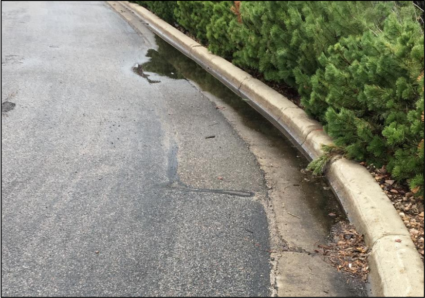
Photo 8. Settled Curb with Ponding Water
