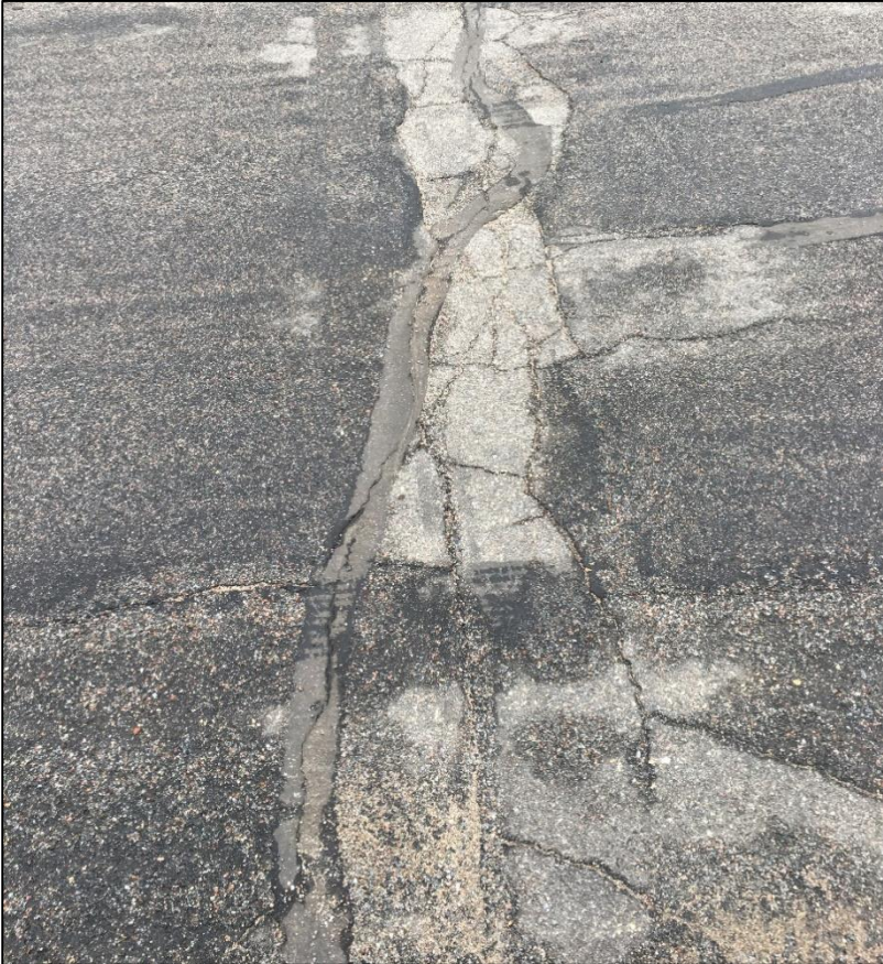
Photo 1. High Severity Transverse Crack Previously Sealed, Victoria Way
