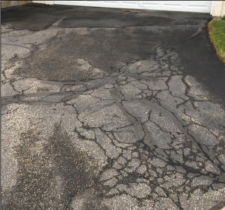
Photo 5. Linear and Alligator Cracks
