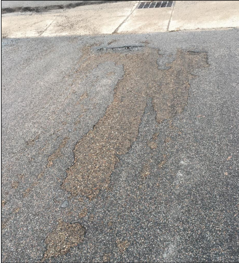
Photo 4. Chip Seal and Surface Delamination, East Entrance to Community
