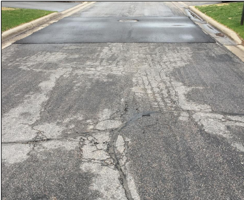
Photo 3. Moderate Severity Alligator Cracking and Large Patch, Southeast end of Victoria Curve
