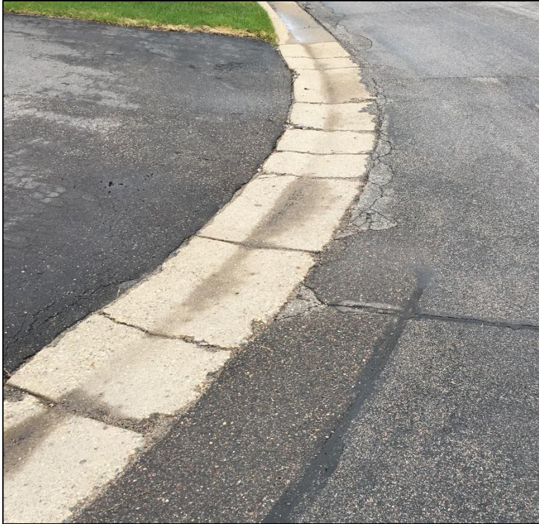
Photo 10. Cracked Interior Curb at Driveway
