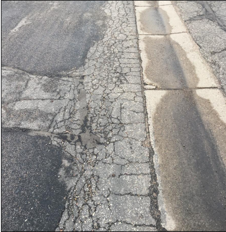
Photo 2. High Severity Edge Cracking, Victoria Curve
