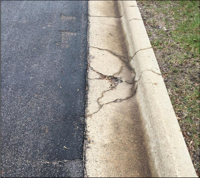
Photo 9. Cracked Exterior Curb
